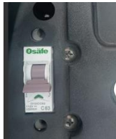
2. MCB is turned OFF
